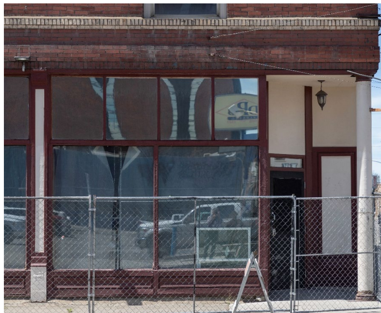
Figure 3. East facade, cast iron post (left edge of photo) and cast iron column (right edge of photo) view.
