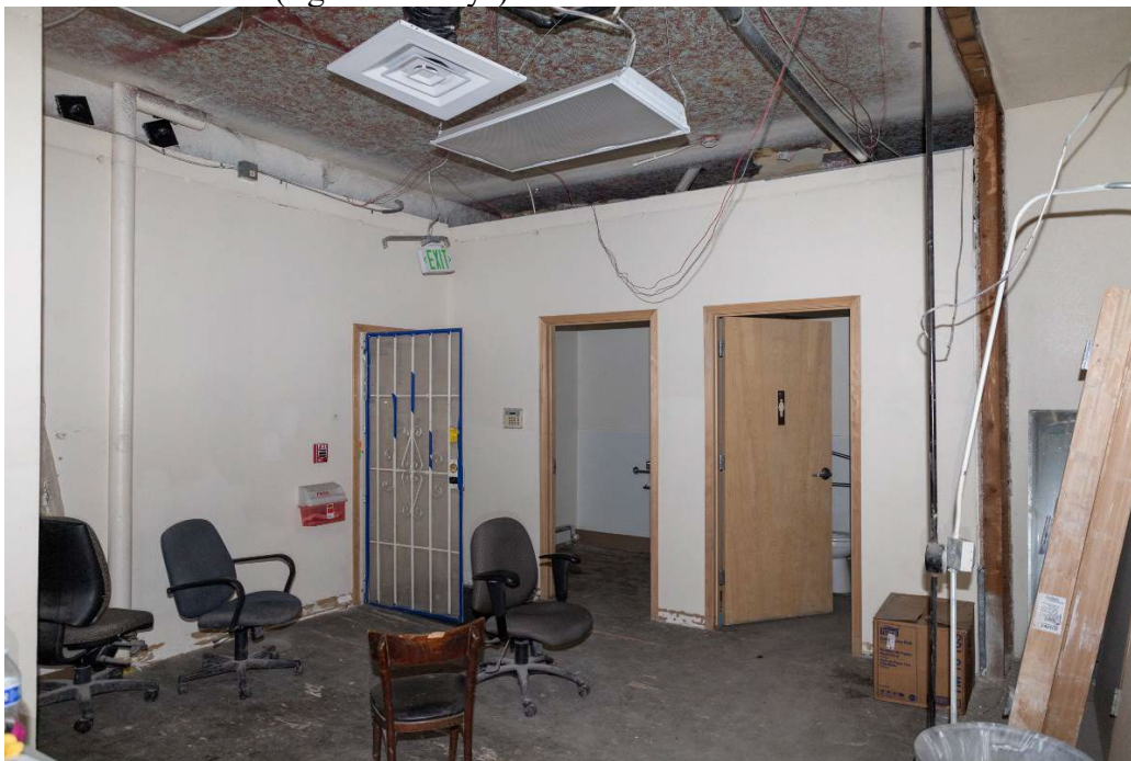
Photo 0021. First floor, looking southeast towards the alley entrance (left doorway) and the two bathrooms (right doorways).
