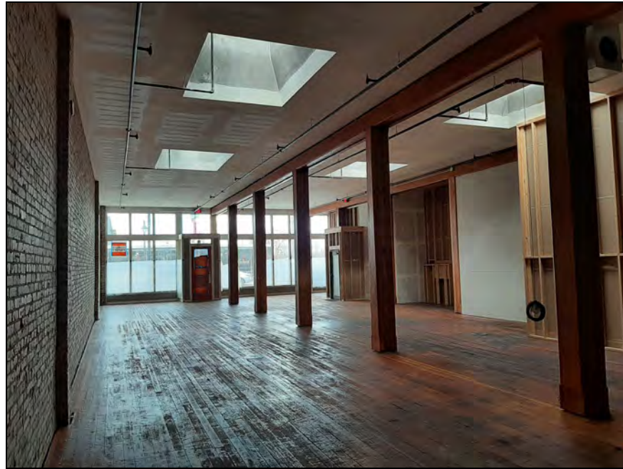
Photo 13 Looking north at the first floor of the attached single-story building at the west elevation of the Framingham Building
