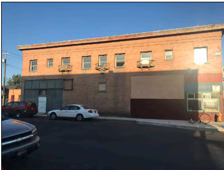
The north façade and east face of the Framingham Building in 2019 before rehabilitation in 2019-2021.
