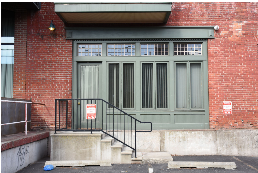
10. South facade-former loading door converted to pedestrian door with windows, looking north
