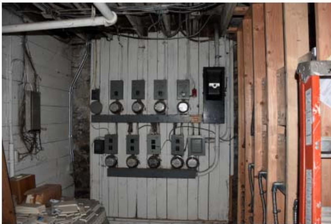
15. Ground floor-electrical panel
