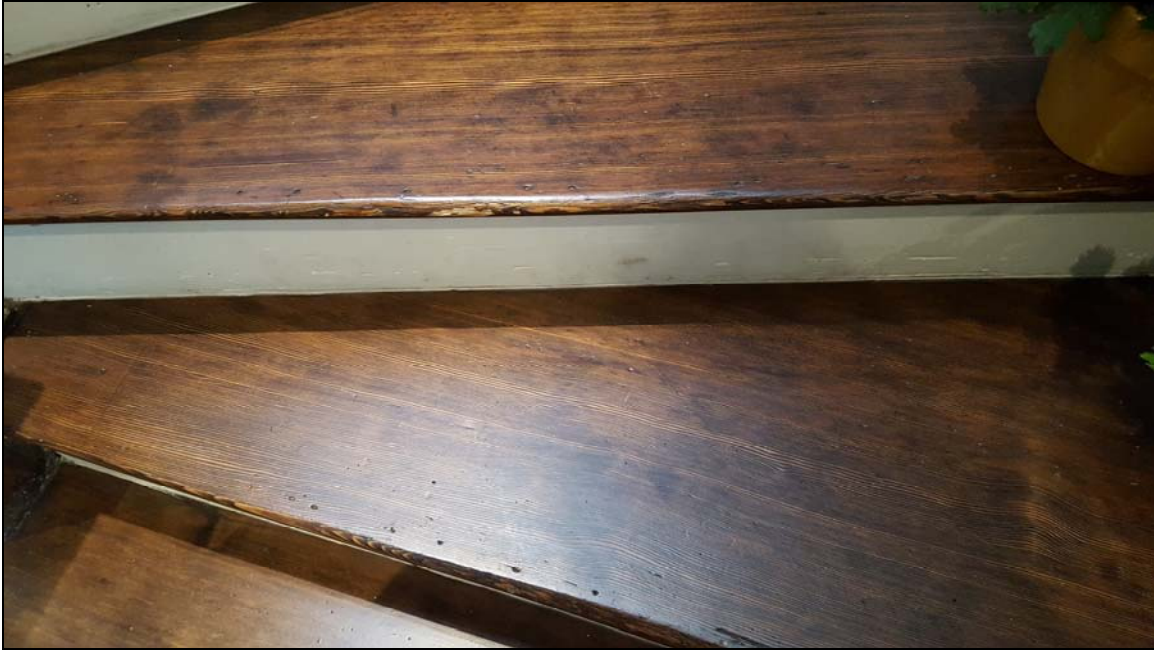
Number 23—stair treads on staircase that rises from first to second floor
