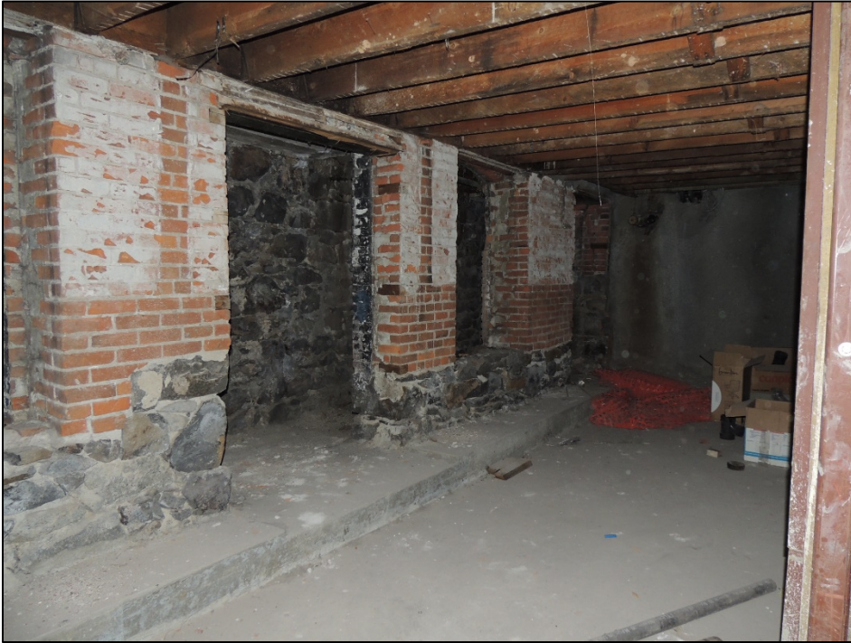
Logan Camporeale, "Interior of basement of south end of building with historic below ground storefront," December 6, 2018, Spokane Historic Preservation Office Photographs.
