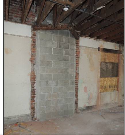
Hotel Aberdeen, (left) 3rd floor hall, (center) 3rd floor north angled doors, (right) 3rd floor removed lightwell 12/6/2018 by Logan Camporeale, SHPO
