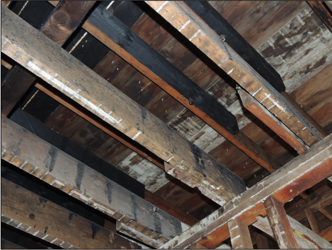
Logan Camporeale, "Third floor rafters showing fire damage and repair," December 6, 2018, Spokane Historic Preservation Office Photographs.
