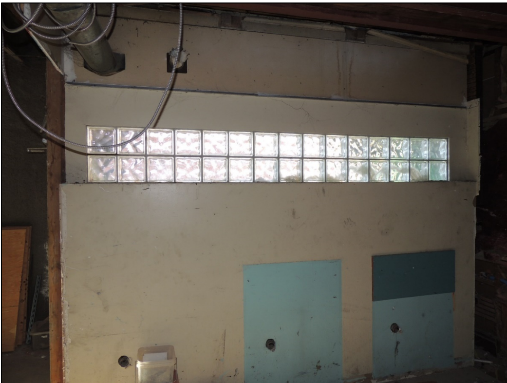
Logan Camporeale, "Area behind main arch entry that was closed in by a previous owner," December 6, 2018, Spokane Historic Preservation Office Photographs.
