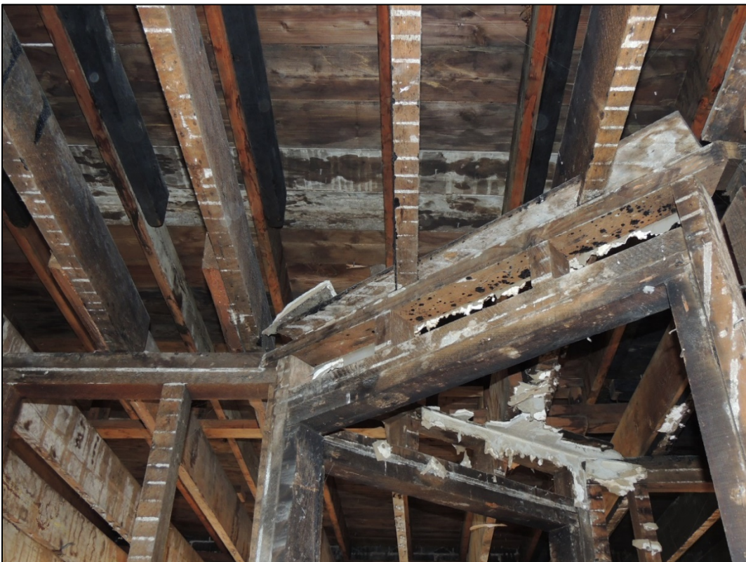
Logan Camporeale, "Third floor rafters showing fire damage and repair," December 6, 2018, Spokane Historic Preservation Office Photographs.
