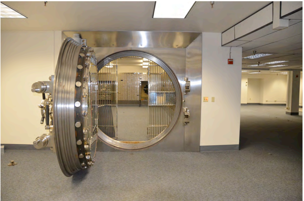
Photo 8 – View to North Showing Vault Door (By Allied Safe & Vault Co of Spokane)
