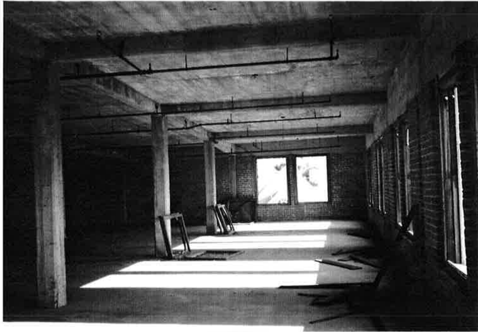
Photos 42, 43 and 44: Third-floor interior looking south; east wall stairtower leading to roof, 1998.
