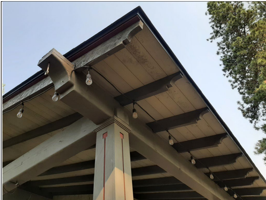
Photo 6 A 2023 photo showing tapered roof eaves at the southeast corner of the front porch
