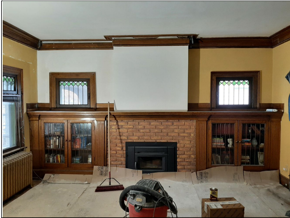
Looking at the west wall of the living room in 2023 during repairs
