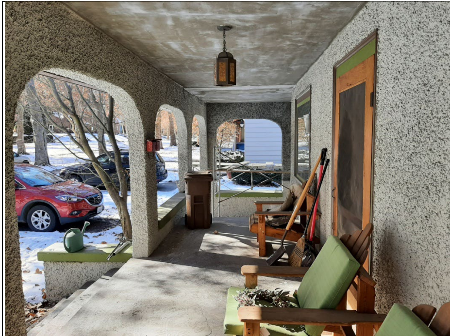
Photo 3 The south facade front porch of the Ritter House, looking west in 2023
