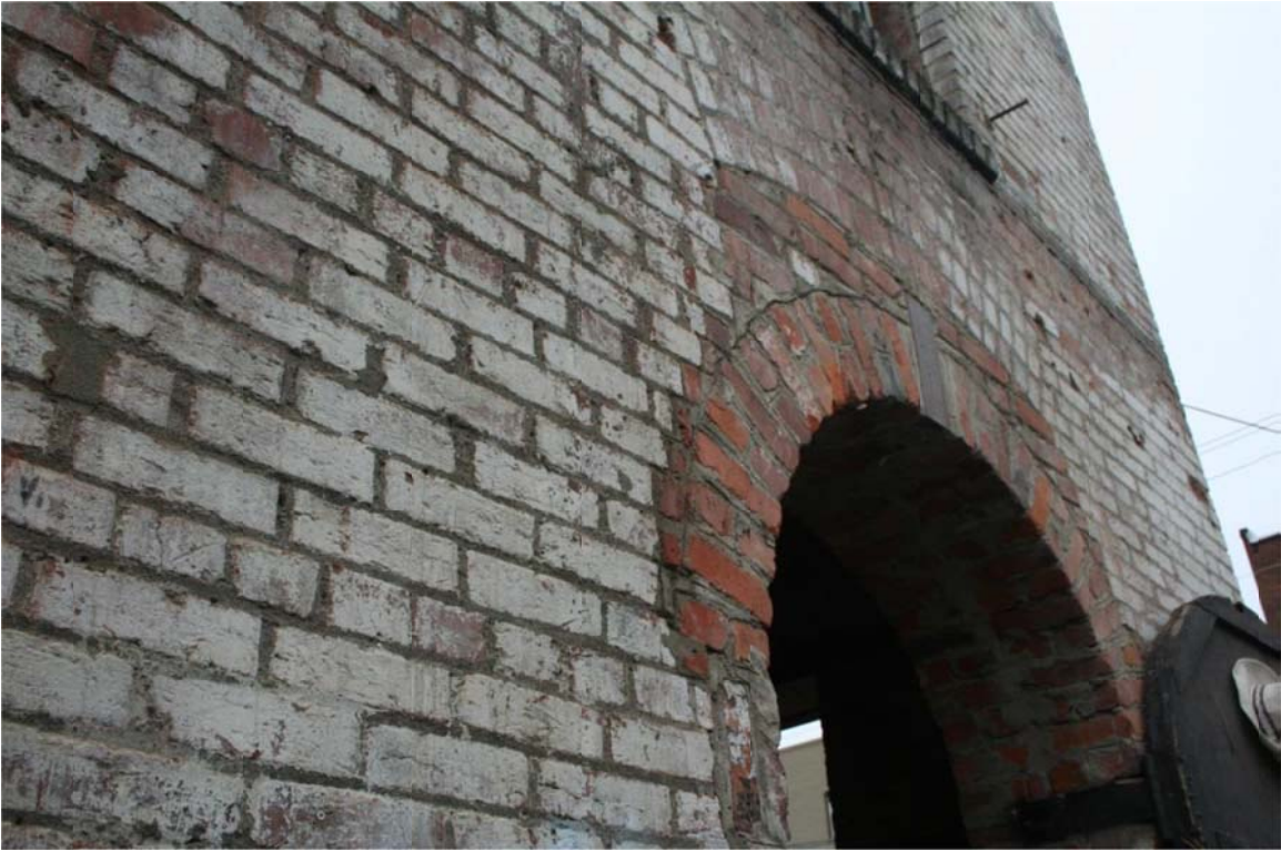
VNH-9 East elevation arches, old above and recent below, view to the northwest.
