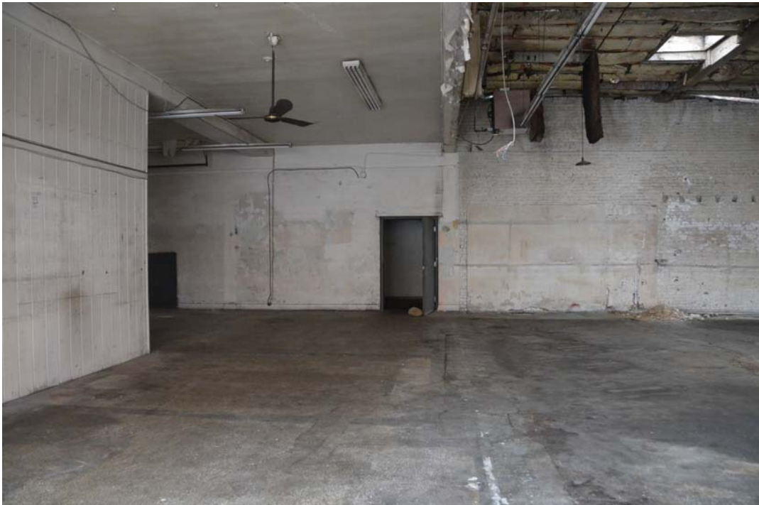
Photo 7 – Looking West Toward West Wall and Door to 1980 Addition (View From Bay 2)
