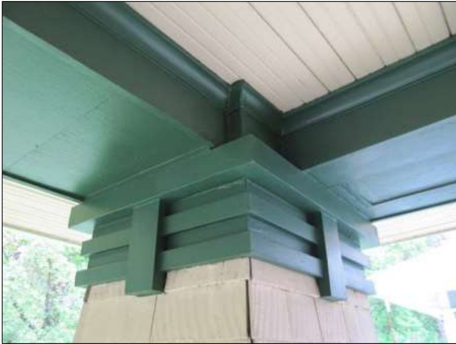
Architectural detail at top of shingled porch pier at front porch in 2015
